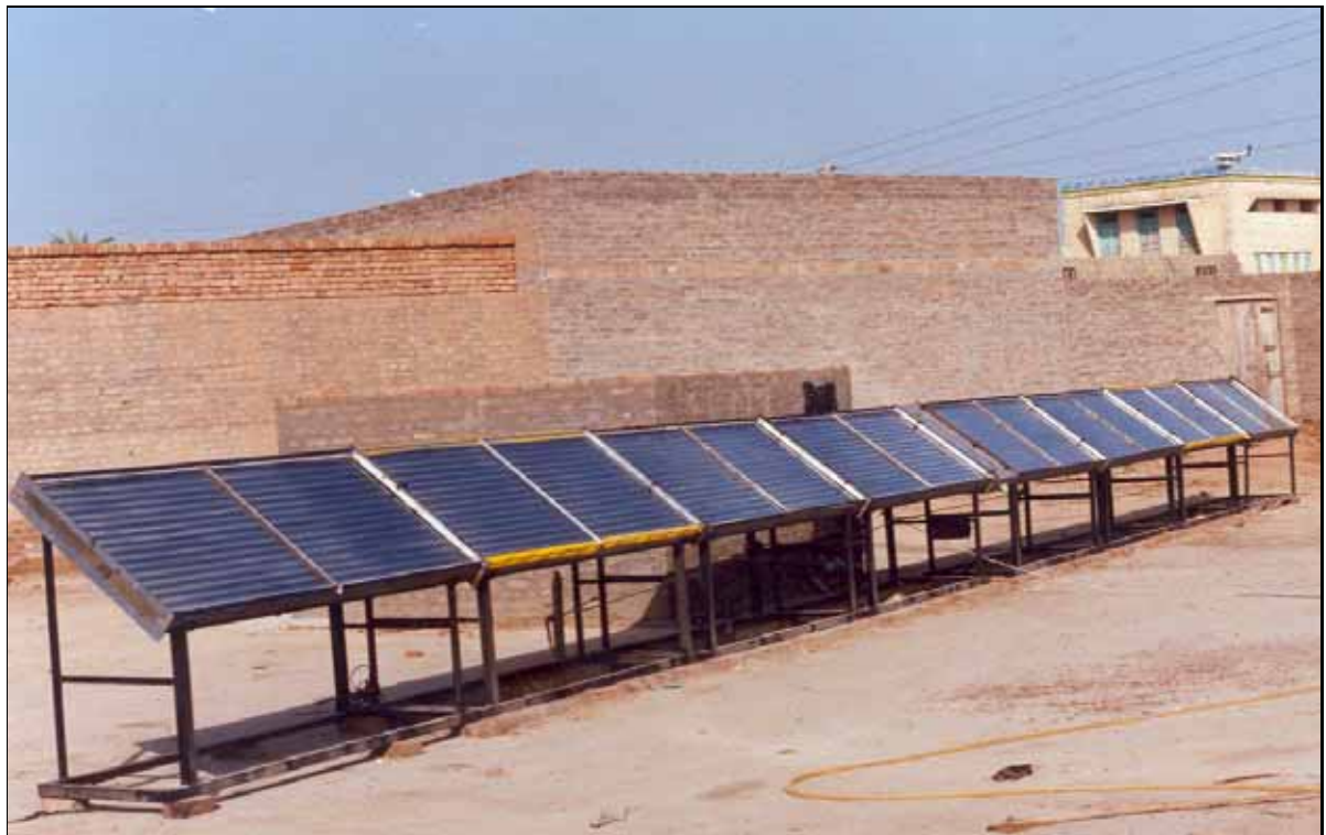
Figure 7: FMI Solar-cum-gas Fired Dates Drying System
